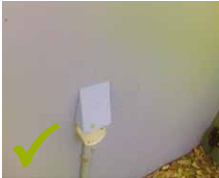
A power outlet has been shielded appropriately.
