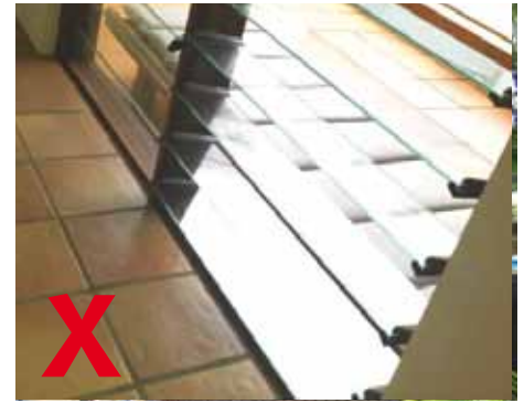
Louvres that create a gap of more than 100 millimetres do not comply.
