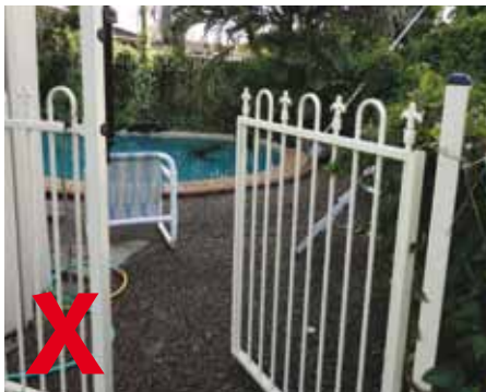
Inward opening gates must be modified to open outwards.
